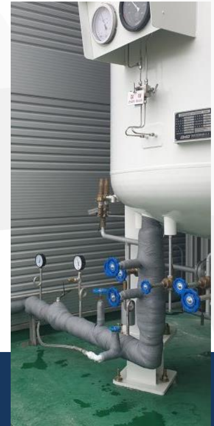
▲ outdoor tanks and Insulation piping line
