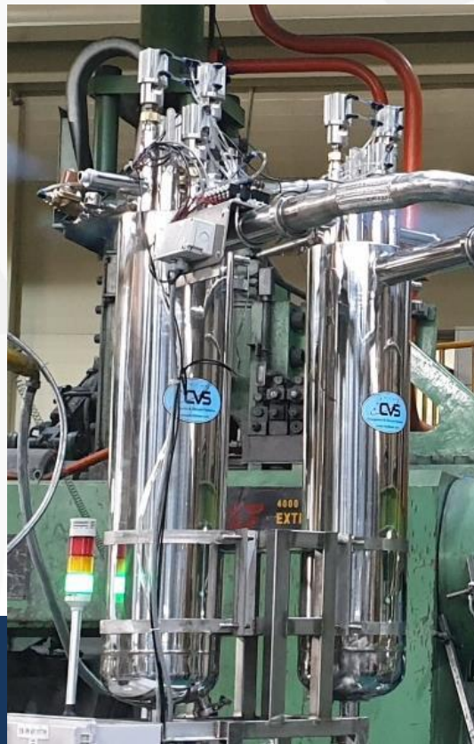
▲ Double Cooling Unit
